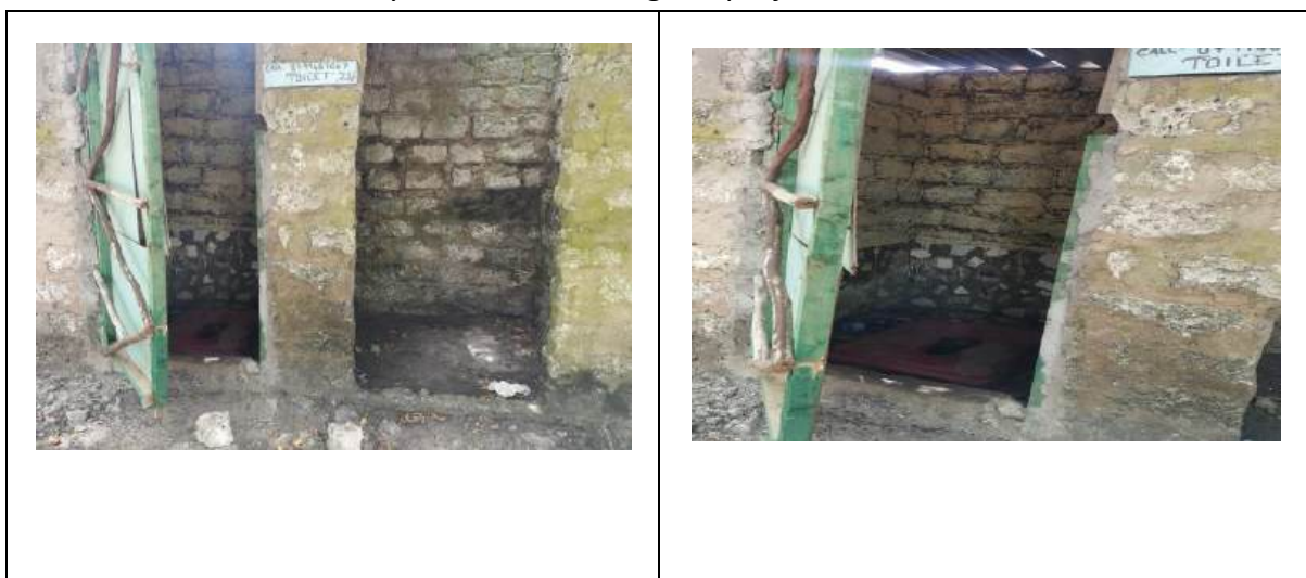
Figure 1: Existing Sanitation Facilities in Mazingira Park
